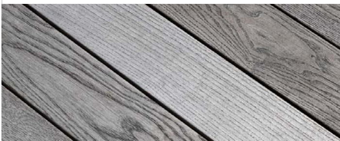
Unoiled Thermory Benchmark thermo-ash decking after 1 year
